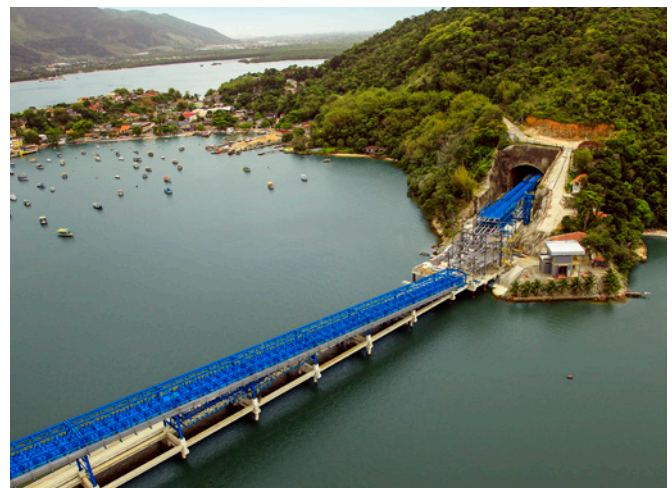
Porto Sudeste iron ore conveyor under construction, Itaguaí, Rio de Janeiro state, Brazil.
